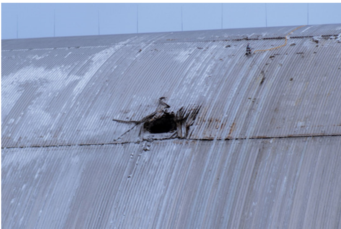
Picture 6: Damaged roof of the new safe confinement at Chornobyl
