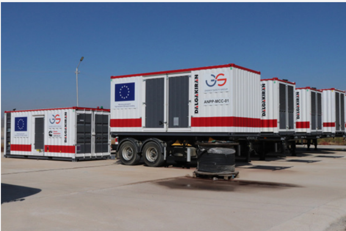
Picture 2: EU-funded equipment – Emergency mobile diesel generators for the Armenian nuclear power plant
