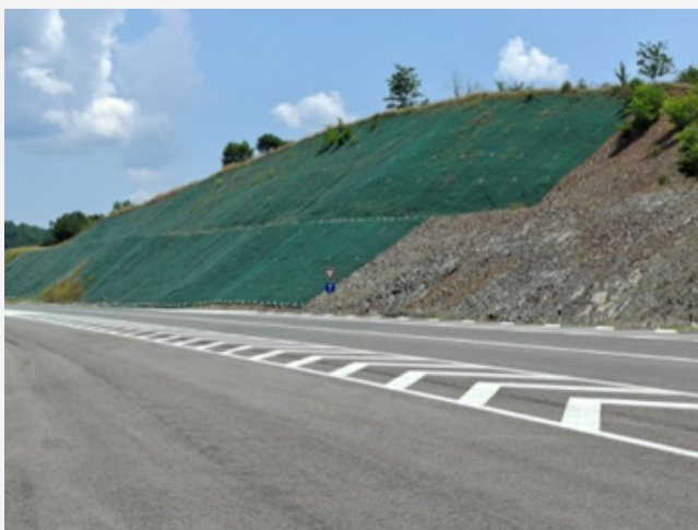
Picture 2 | Slope protected by a stabilisation net
