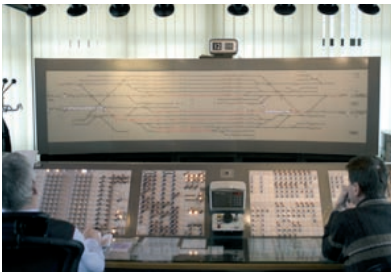
Photo 7 – Traffic control facility at Brennersee station
