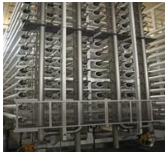
Picture 2: Desalination plant in Spain
