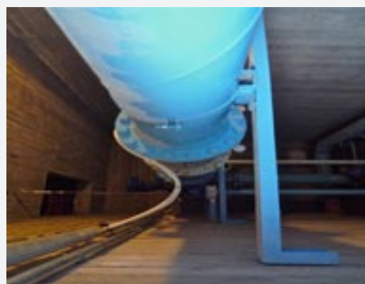
Picture 8: Water transport infrastructure (type B)
