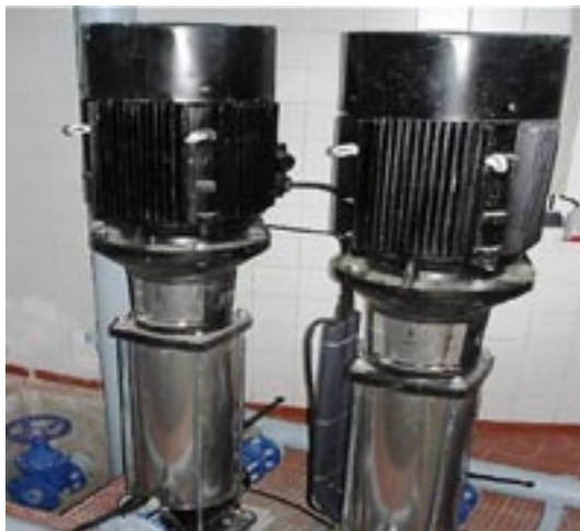
Picture 1: Pumping station in Portugal
