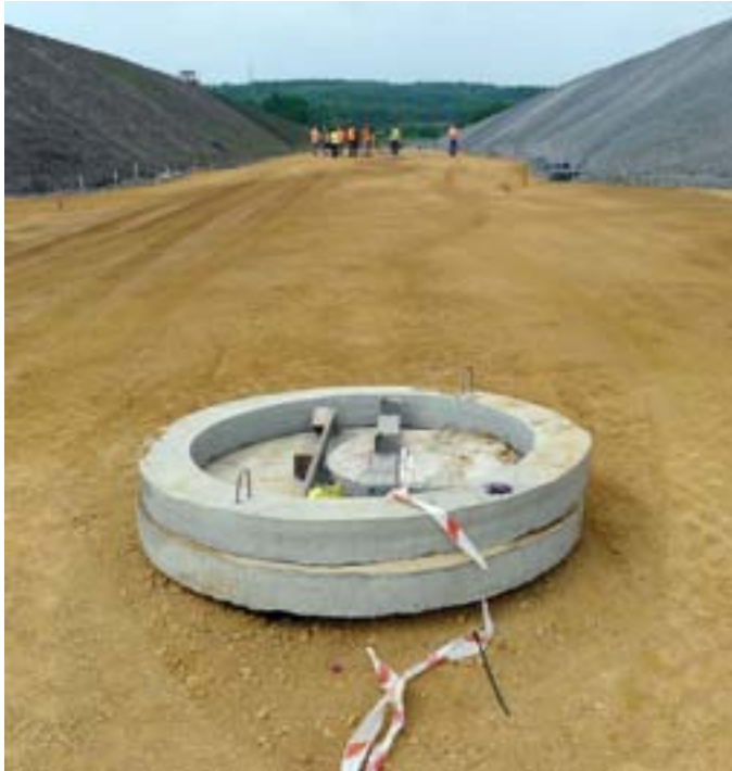
Photo 4 — Roads and utility installations being constructed on the site of a former coal mine slag heaps (Jaworzno, Poland)
