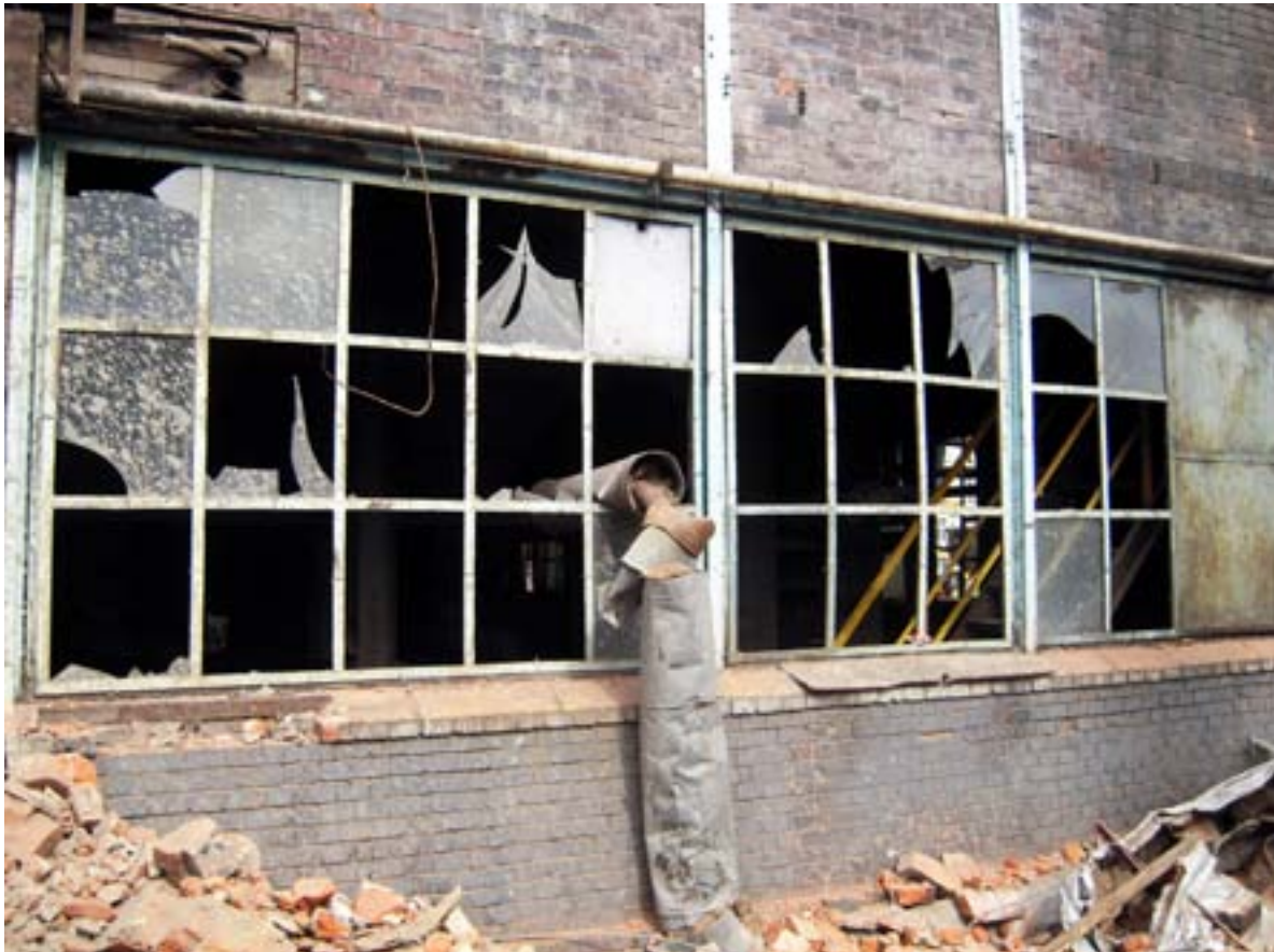
Photo 8 — Old buildings being demolished and renovated at a derelict power station that is being converted into an arts and cultural centre (Łódź, Poland)
